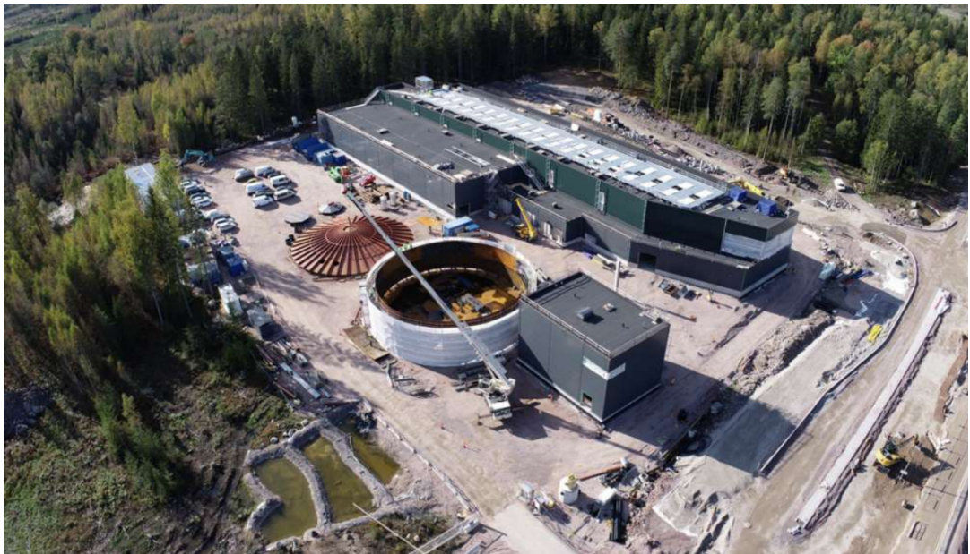
Figure 3: Heat pump station at Kirkkonummi data center (October 2024)
